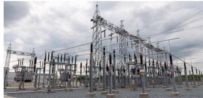
Example of a typical substation
