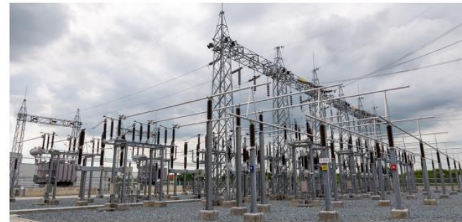
Example of a typical substation
