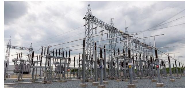
Example of a typical substation
